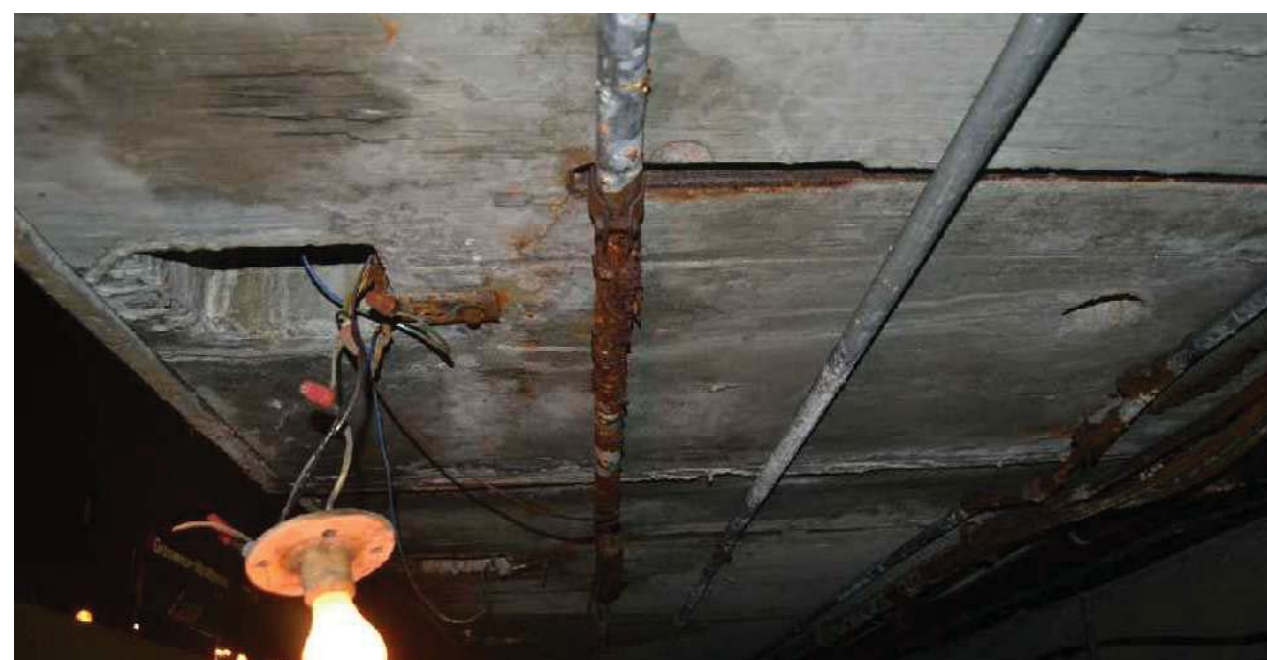
CORRODED CONDUIT DETAIL: PHOTO D A11E-100 SCALE: NOT TO SCALE
