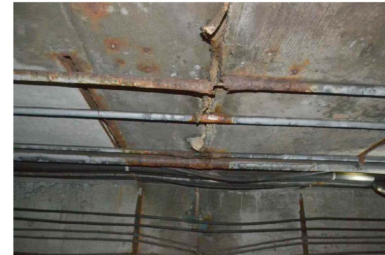
CORRODED CONDUIT DETAIL: PHOTO C A11E-100 SCALE: NOT TO SCALE
