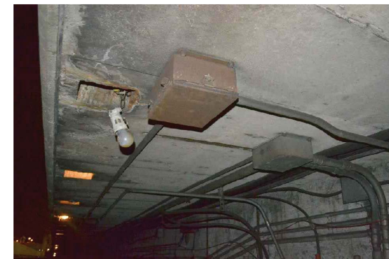
CORRODED PULL BOX DETAIL: PHOTO F A11E-100 SCALE: NOT TO SCALE
