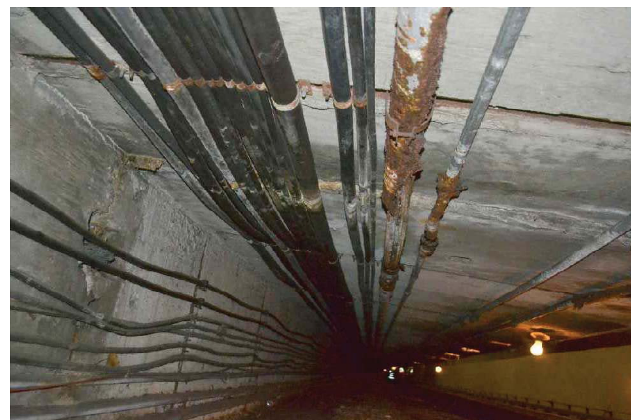
CORRODED CONDUIT DETAIL: PHOTO E A11E-100 SCALE: NOT TO SCALE
