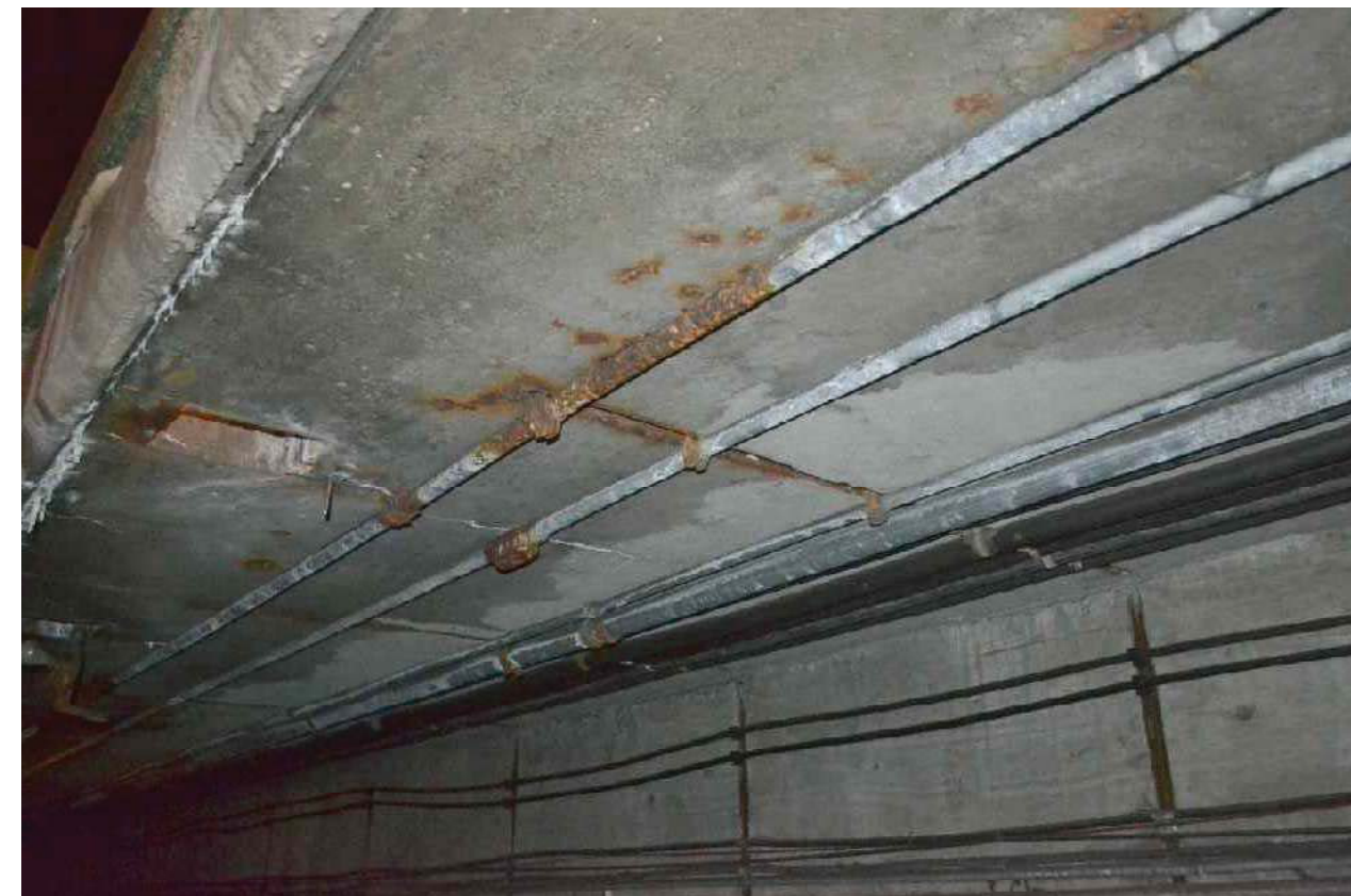
CORRODED CONDUIT DETAIL: PHOTO B A11E-100 SCALE: NOT TO SCALE
